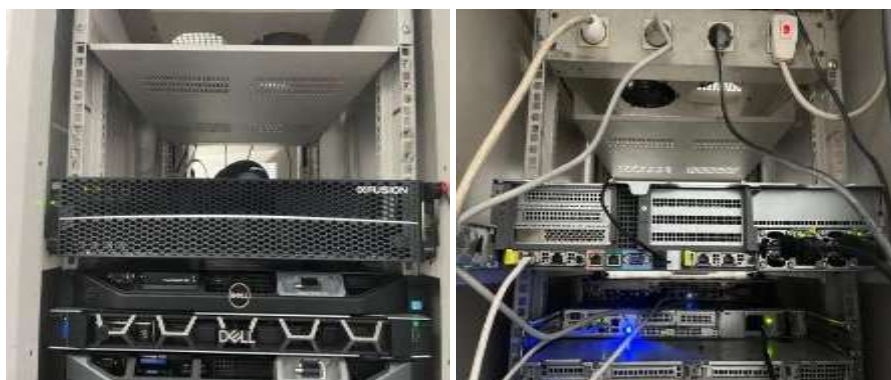
Gambar 3. 7 Server x fusion terpasang
